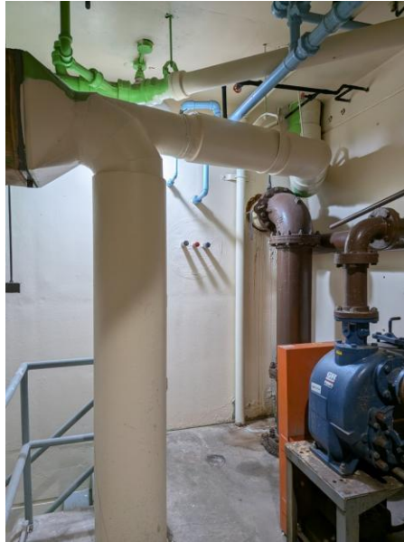
Transite piping on 1 st basement level.
